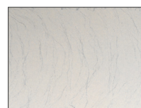
COVERAGE TOO LIGHT
